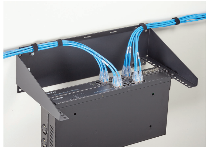
Figure 1. Equipment installed on RMT052-R2 bracket mounted on a wall.
