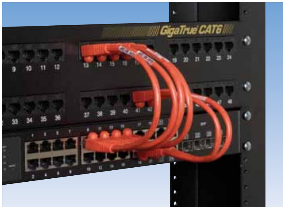
Shown: CAT6 Reduced-Length Cable (EVNSL643-006IN) connecting our GigaTrue® CAT6 48-Port Patch Panel (JPM612A-R6), blackbox.com with the 24-Port Managed Back Office Switch (LGB2003A-R2), blackbox.com
