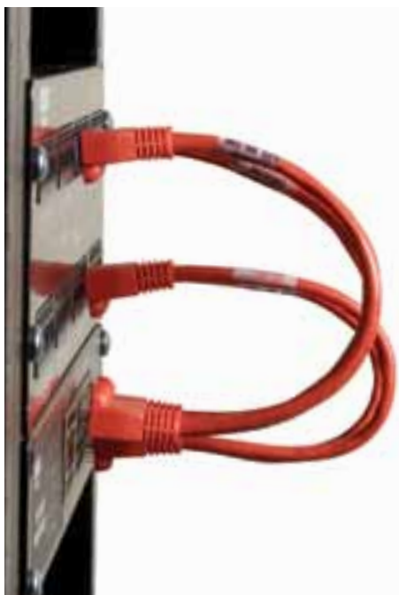
No need for horizontal cable management.
