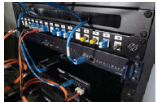
SmartPath EMS Appliance (LWN600MA) installed in a data centre.
